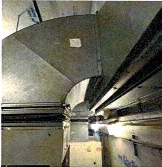
Figure 4. VRV condensers discharge is located in a common exhaust plenum.
