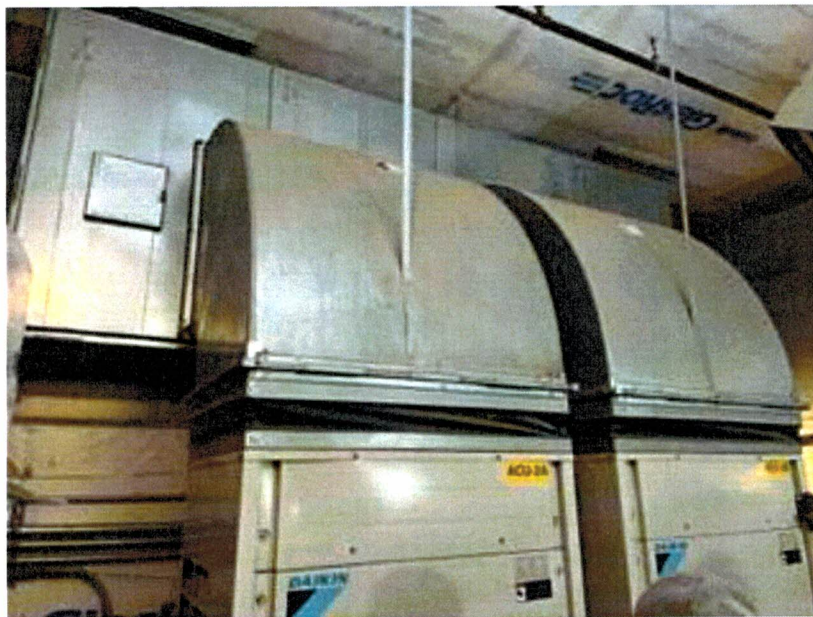
Figure 3. Discharge air from VRV condensers ducted to exhaust plenum and louver.
