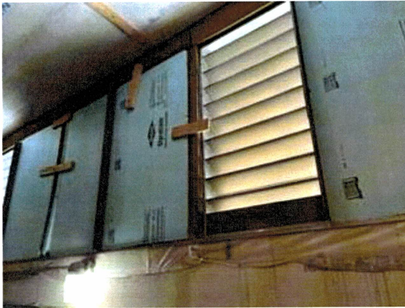
Figure 2. Intake louver in the penthouse. Note that portions of the intake louver have rigid insulation blocking sections of louver off.
