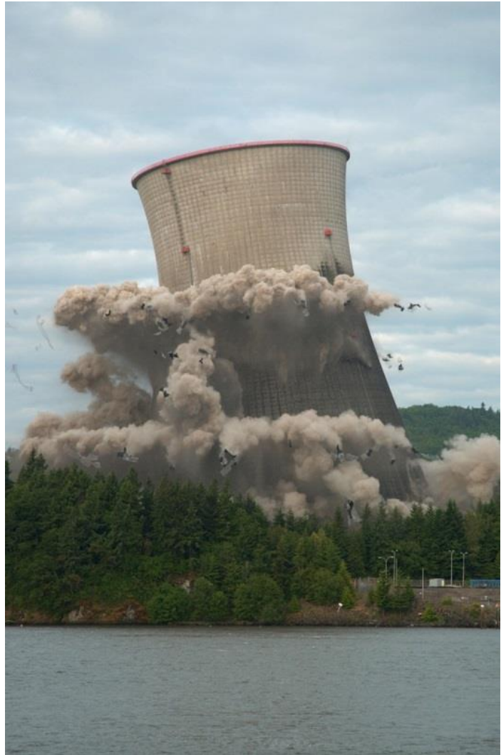
The Trojan cooling tower was imploded on May 21, 2006. Because the tower was visible from I-5, PGE closely coordinated with ODOT and the Highway Patrol to conduct a rolling slowdown of traffic prior to the implosion, so drivers who were unaware of the planned explosion were not alarmed, causing an accident.
