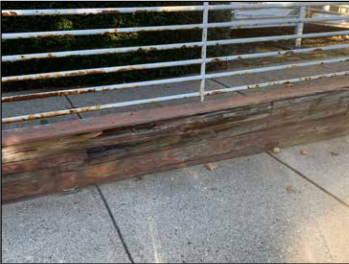
Image 4: Existing railing and wood retaining wall with rotting boards along sidewalk.
