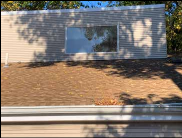
Image 46: View of roof with shingles in need of repair / replacement.
