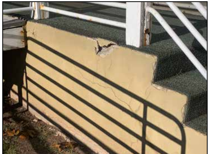
Image 7: Existing railing with cracking and damage.
