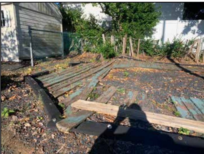
Image 56: View of damaged formering playground area.
