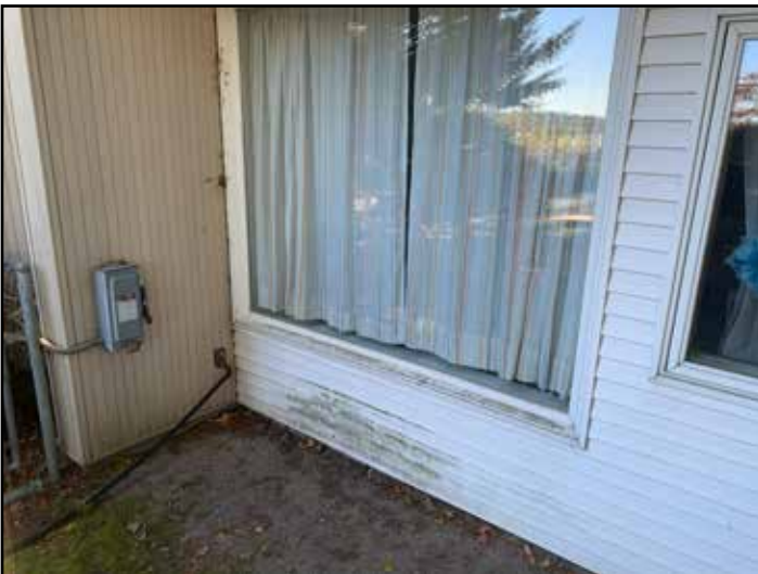
Image 62: View of damaged and molded window and siding.
