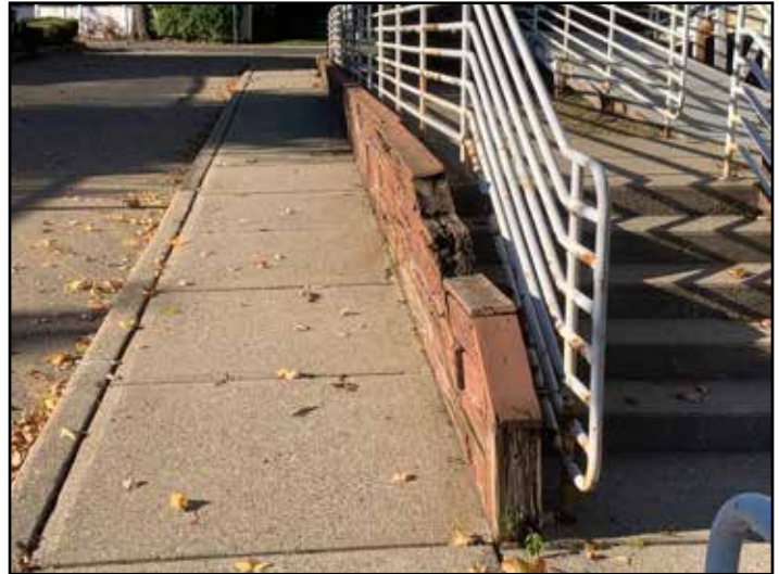
Image 5: Existing railing and wood retaining wall with rotting boards along sidewalk.
