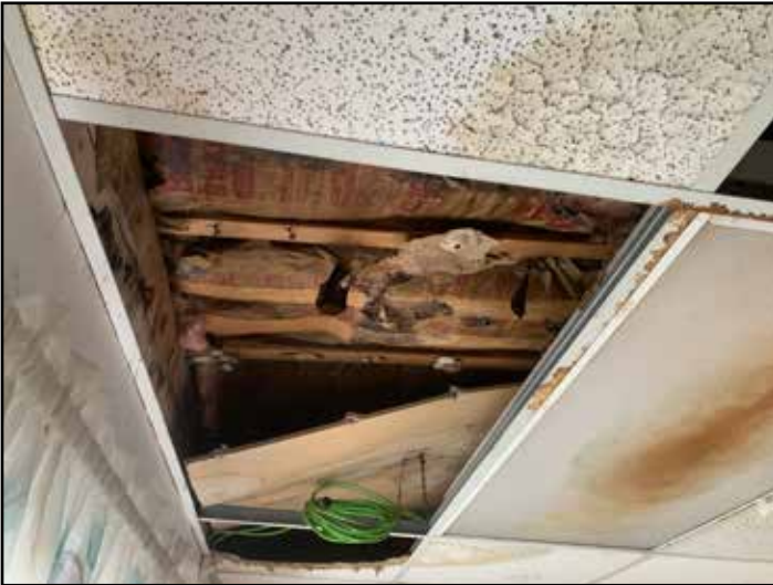
Image 10: Close up of water damage of ceiling tiles.
