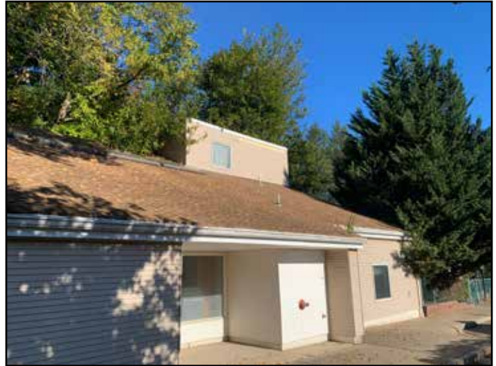
Image 47: View of roof with shingles in need of repair / replacement.
