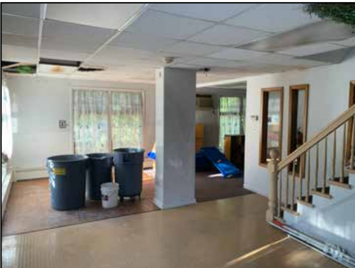
Image 8: Interior former day care with water damage to ceiling tiles
