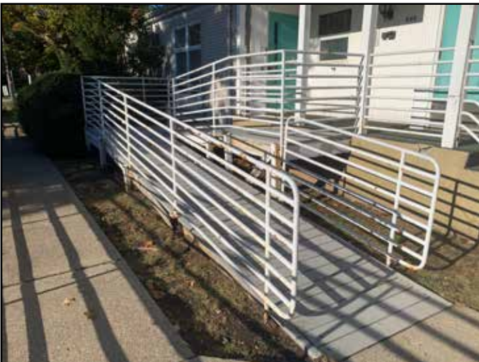
Image 6: Existing railing and wood planks and wall with rotting boards along sidewalk.
