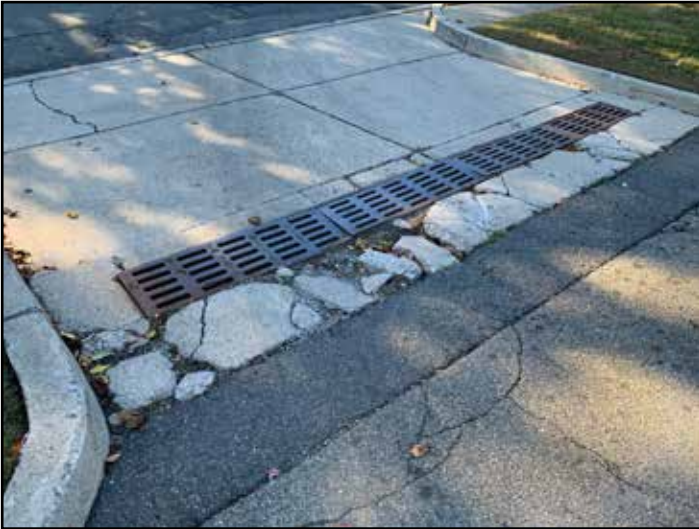
Image 52: View of driveway apron with damage at Windsor Place entrance.
