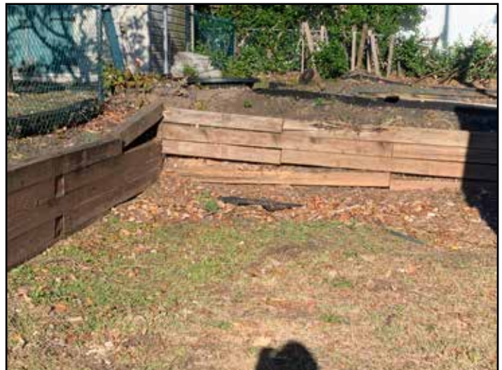
Image 55: View of damaged formering playground area.
