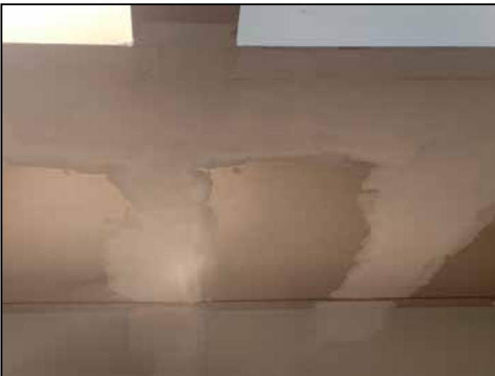
Image 36: Second level ceiling with painted repairs.
