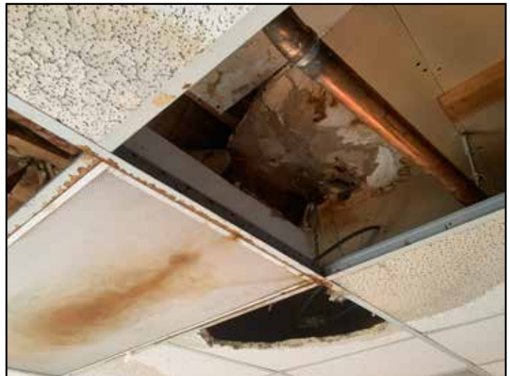
Image 9: Close up of water damage of ceiling tiles.
