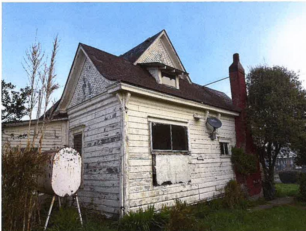
Figure 8 – South Exterior with Damaged Siding and replaced Windows
