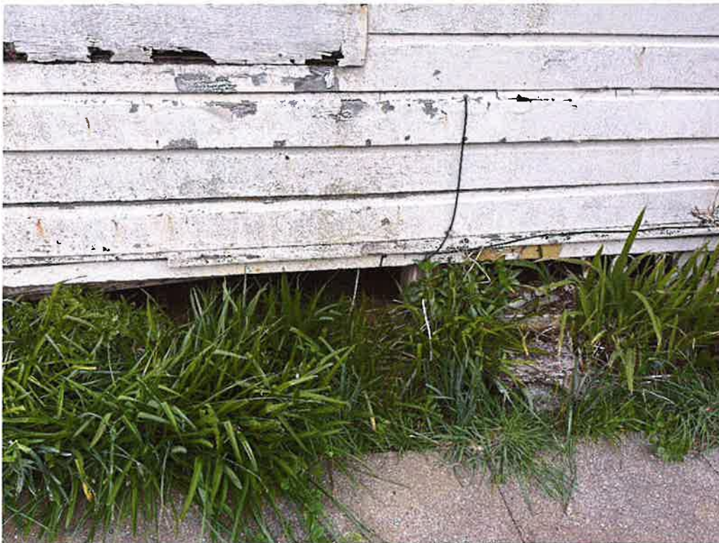
Figure 10 – Wood Post & Pier Foundation with Significant Dry-rot
