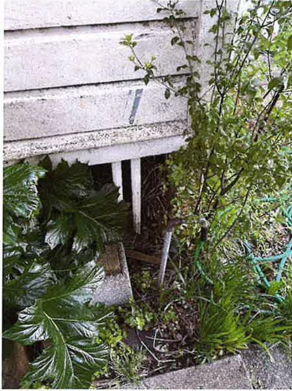
Figure 11 – Southwest Corner Foundation with Significant Dry-rot
