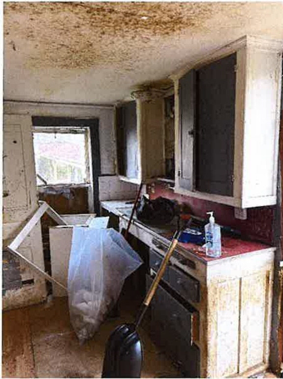
Figure 5 – Kitchen Area with Extensive water Damage and Mold
