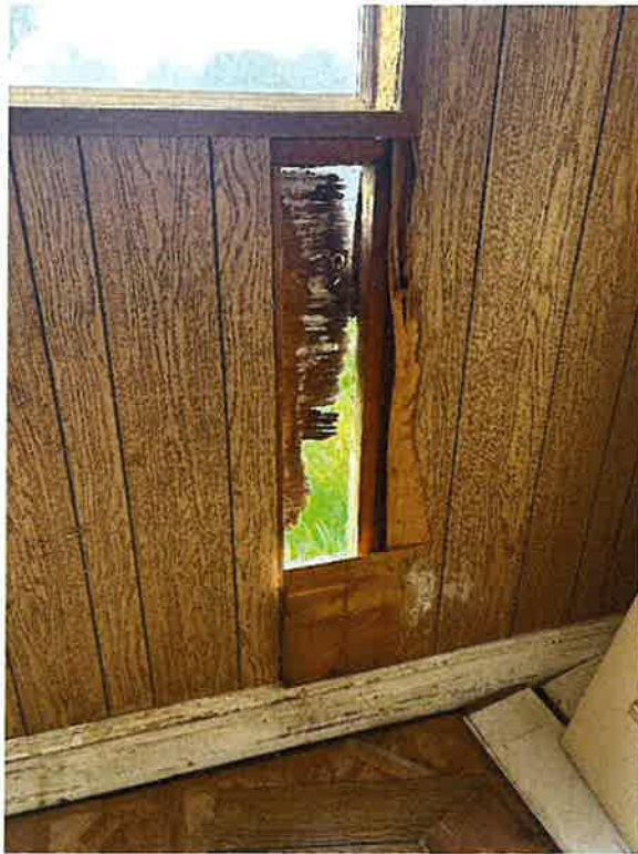
Figure 3 – Dry rot damage in South Exterior Wall
