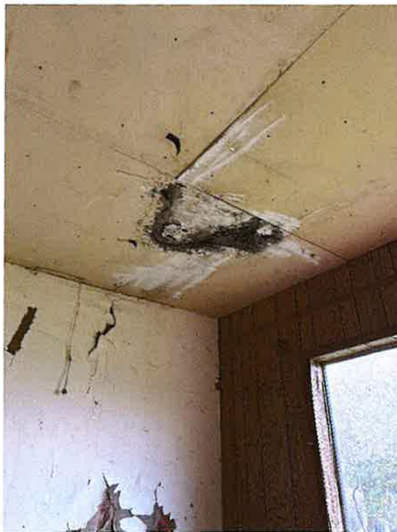
Figure 4 – Mold and Water Damage in Ceiling
