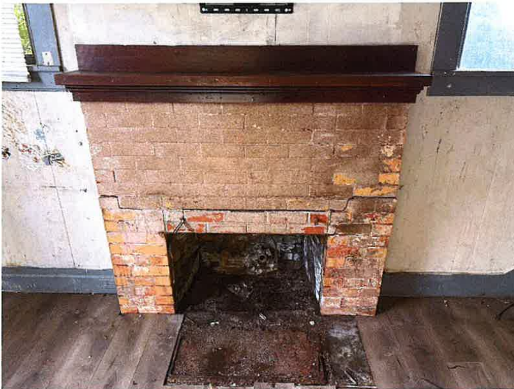
Figure 2 – Settling Masonry Fireplace
