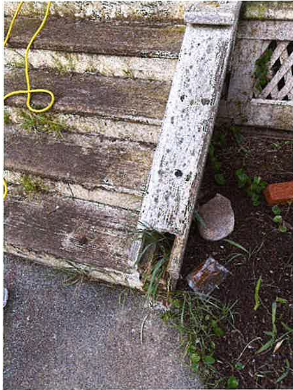
Figure 1 - Dry rot steps and missing handrails on Front Porch
