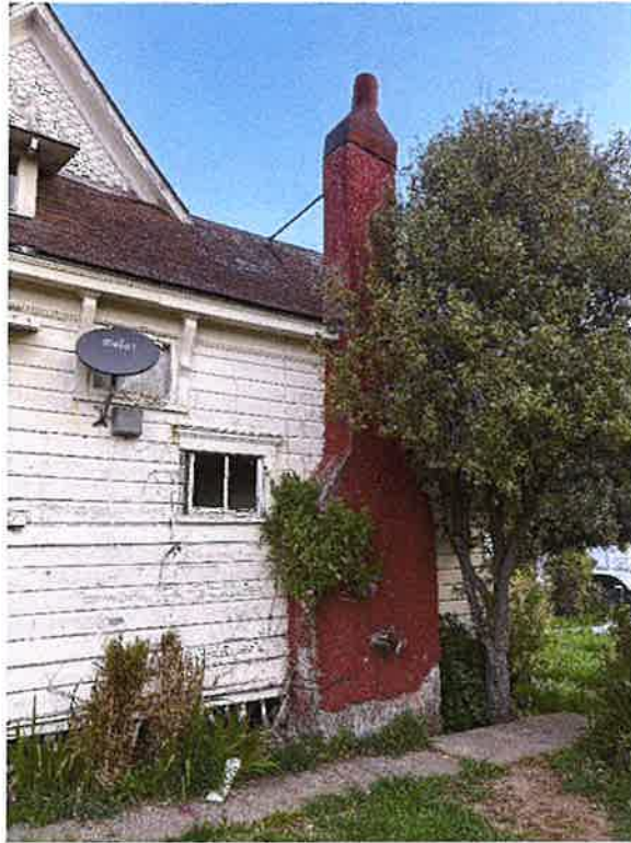
Figure 9 – South Exterior at Fireplace with Damaged Siding
