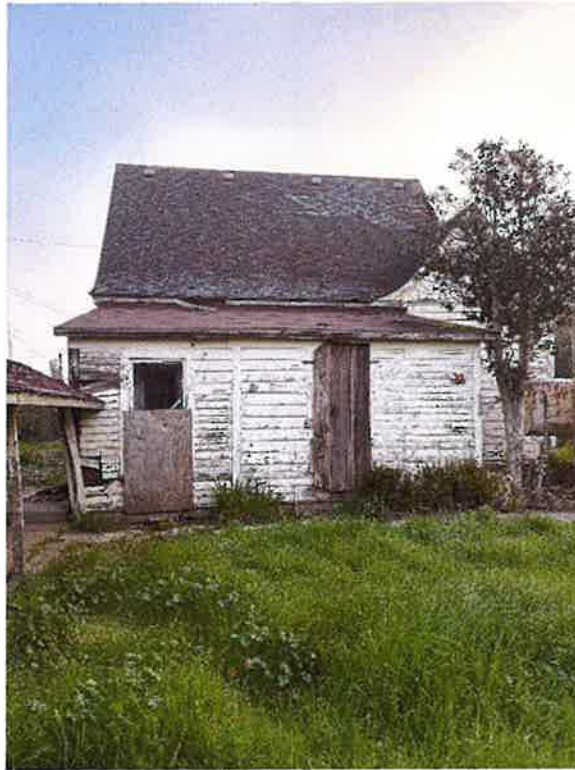
Figure 7 – West Exterior with Kitchen Addition. Note Roof Disrepair.
