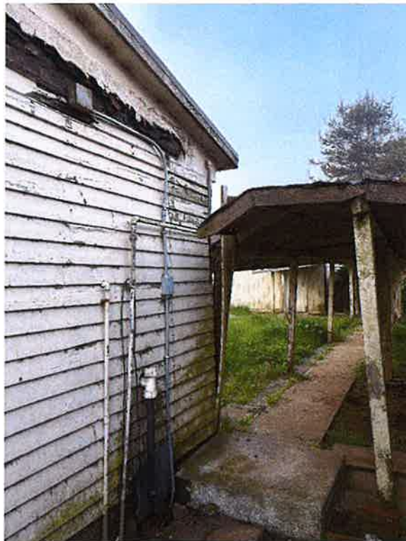
Figure 6 – North Exterior. Note Missing Awning and Damaged Siding
