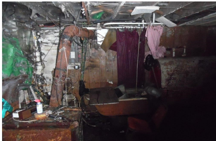
938 Shank Road—Interior Condemnation
