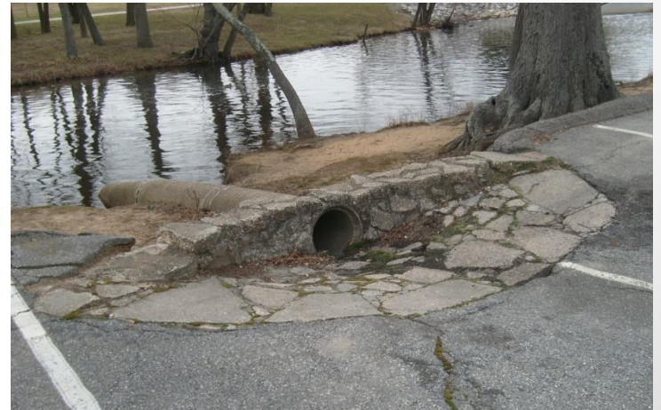
Picture of direct discharge of stormwater into the St. Jones
