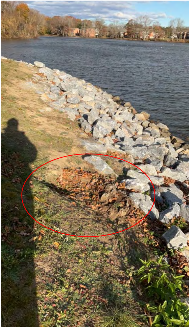
PHOTO 15: Right embankment upstream slope. Erosion/settlement at dead stump.
