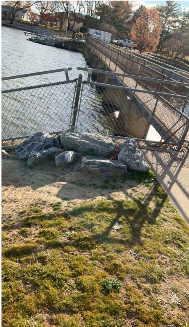
PHOTO 14: Bare earth and minor erosion on upstream embankment slope at right spillway wingwall.
