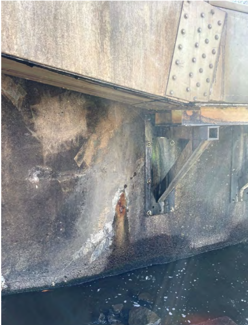
PHOTO 57: Closeup of third seep at crack/former attachment point. Rust staining noted.
