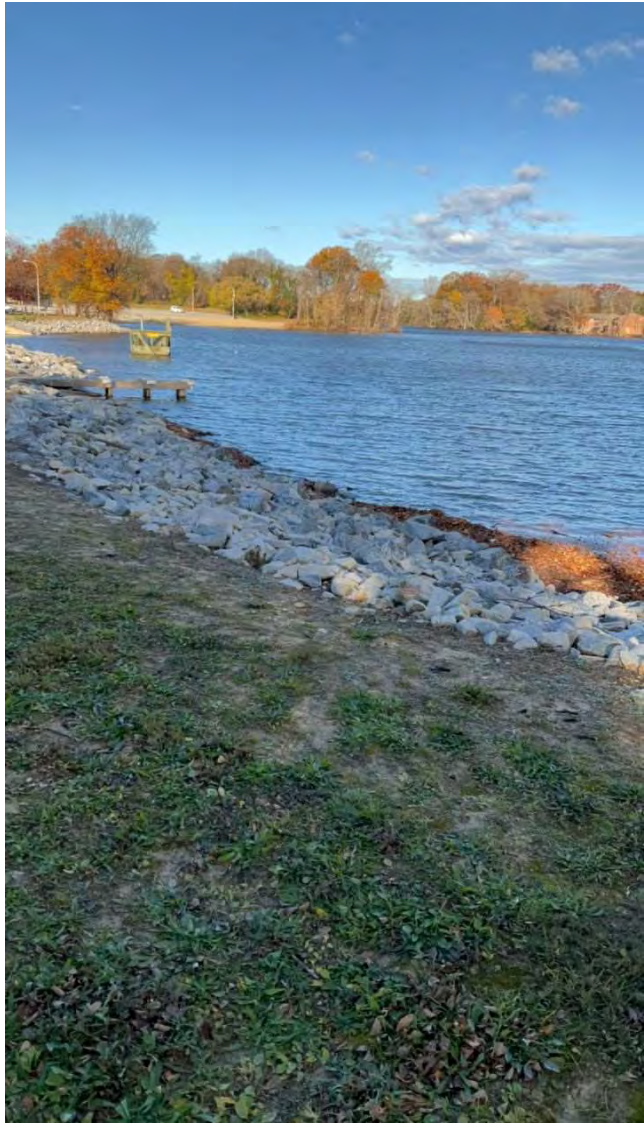
PHOTO 2: Left embankment upstream slope. Bare area above riprap armor.
