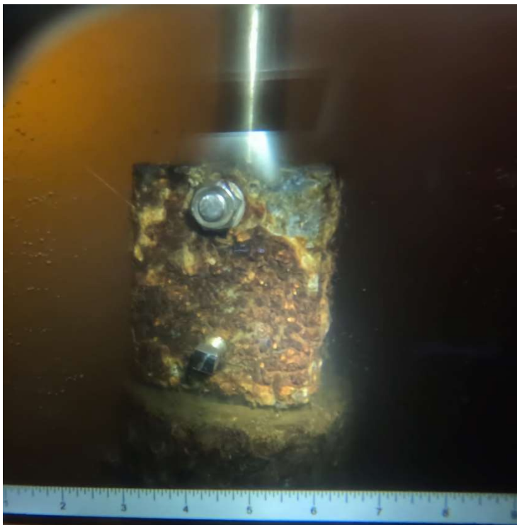
PHOTO 5: Gate stem coupler and gate stop
