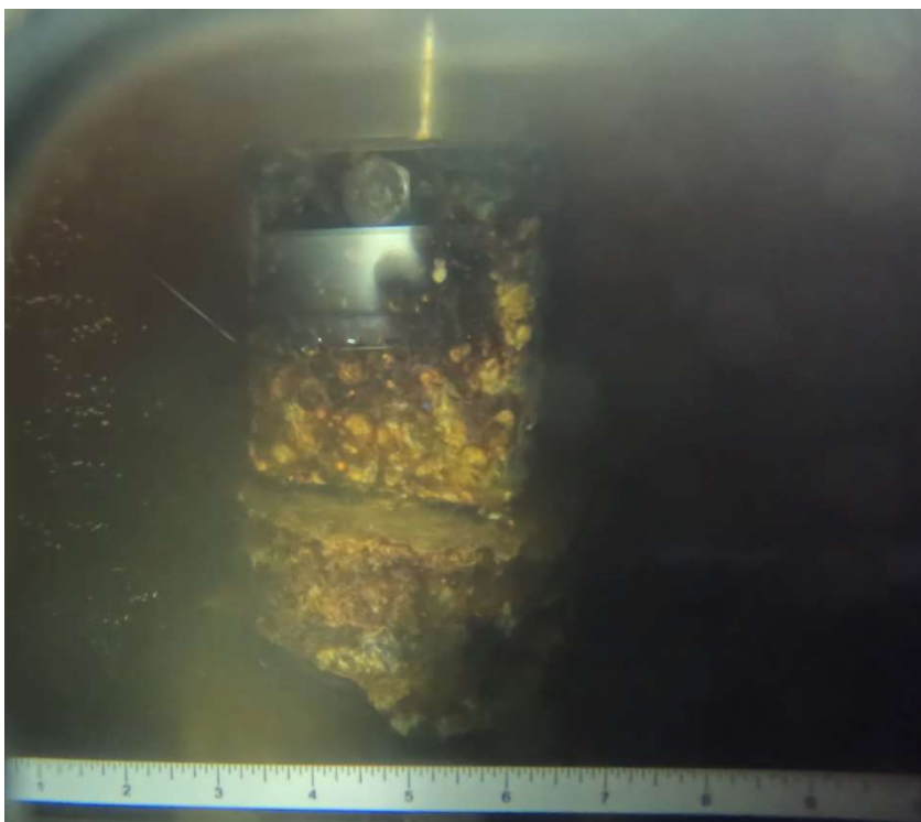
PHOTO 6: Gate stem coupler and gate stop
