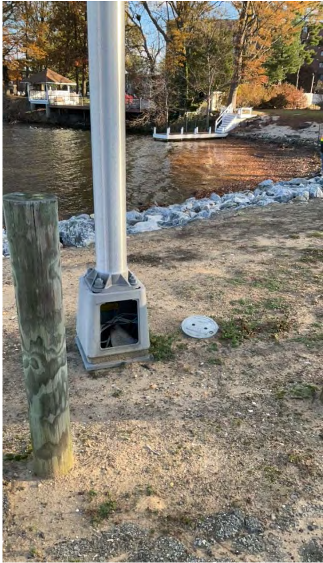
PHOTO 4: Open access panel and exposed wiring at light in embankment. Bare earth above riprap
