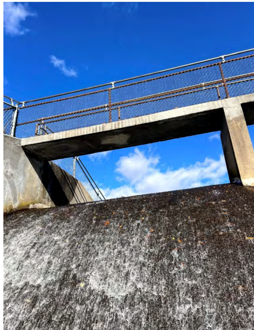
PHOTO 44: Typical condition, underside of pedestrian access bridge deck.
