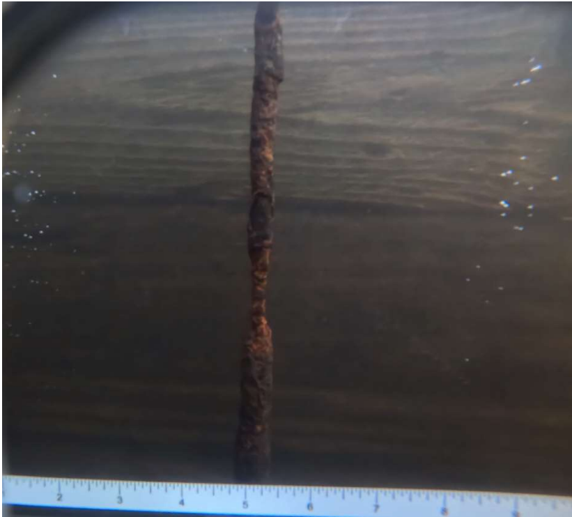
PHOTO 19: Vertical trash rack rod below waterline
