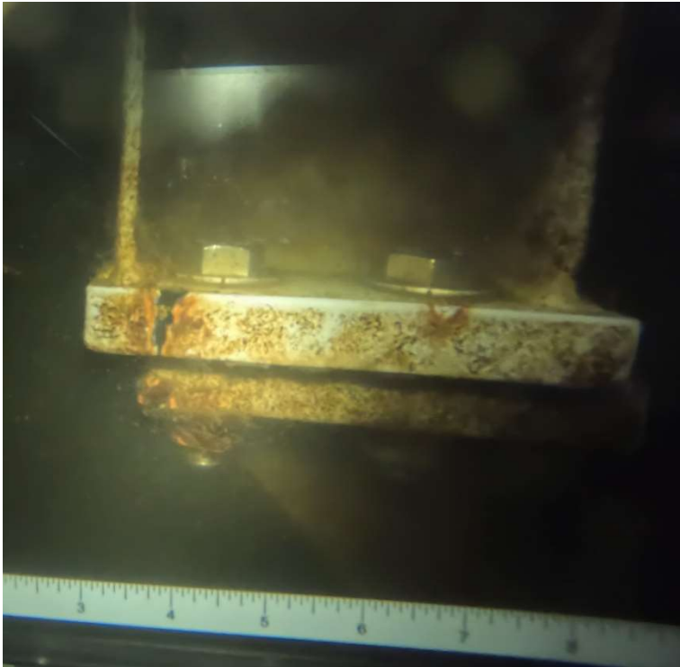
PHOTO 9: Gate frame connection
