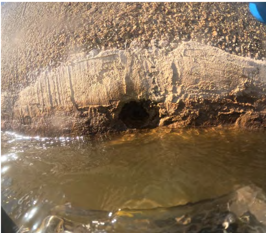
PHOTO 24: Prior concrete repair at right training wall
