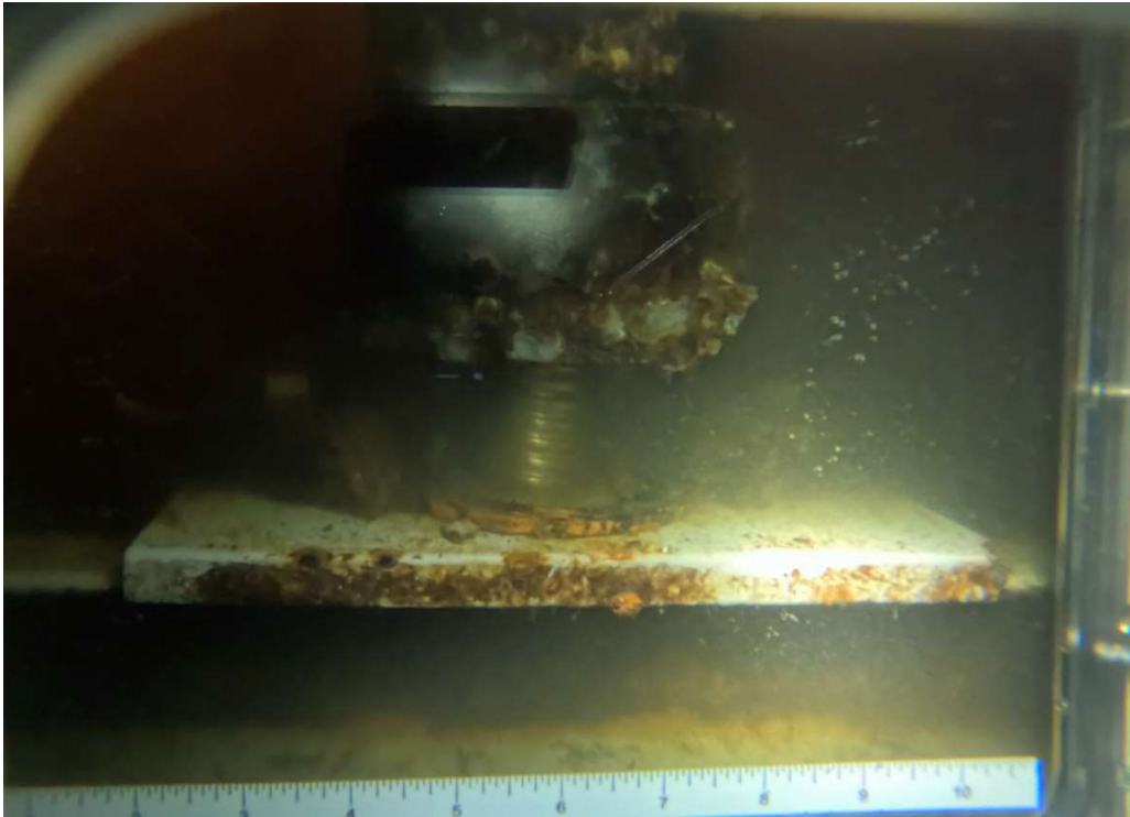
PHOTO 7: Gate stem coupler and gate stop
