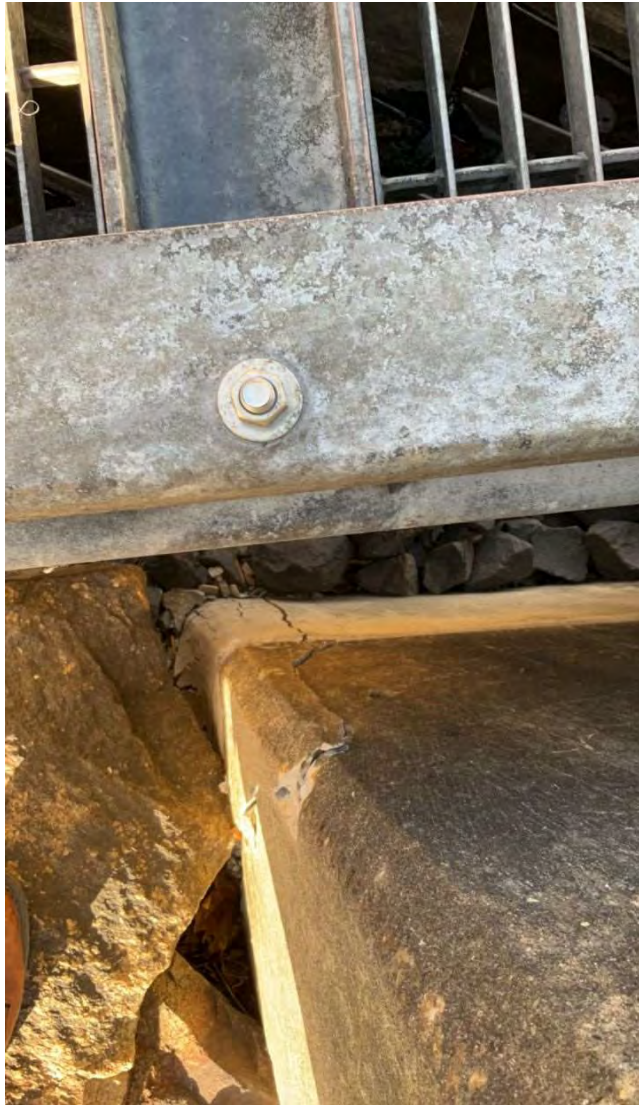
PHOTO 30: Damage at downstream end of left spillway wingwall, adjacent to fish ladder.
