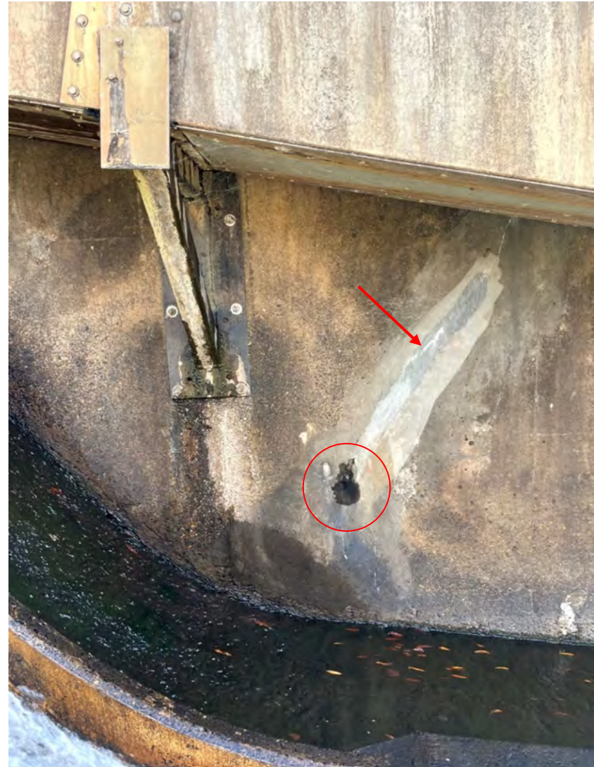
PHOTO 56: Prior crack repair used flexible sealant on top of concrete/mortar patch indicated by arrow.
