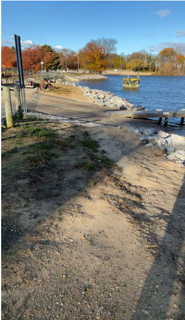
PHOTO 5: Bare earth and minor erosion along upstream slope of left embankment approaching boat ramp.
