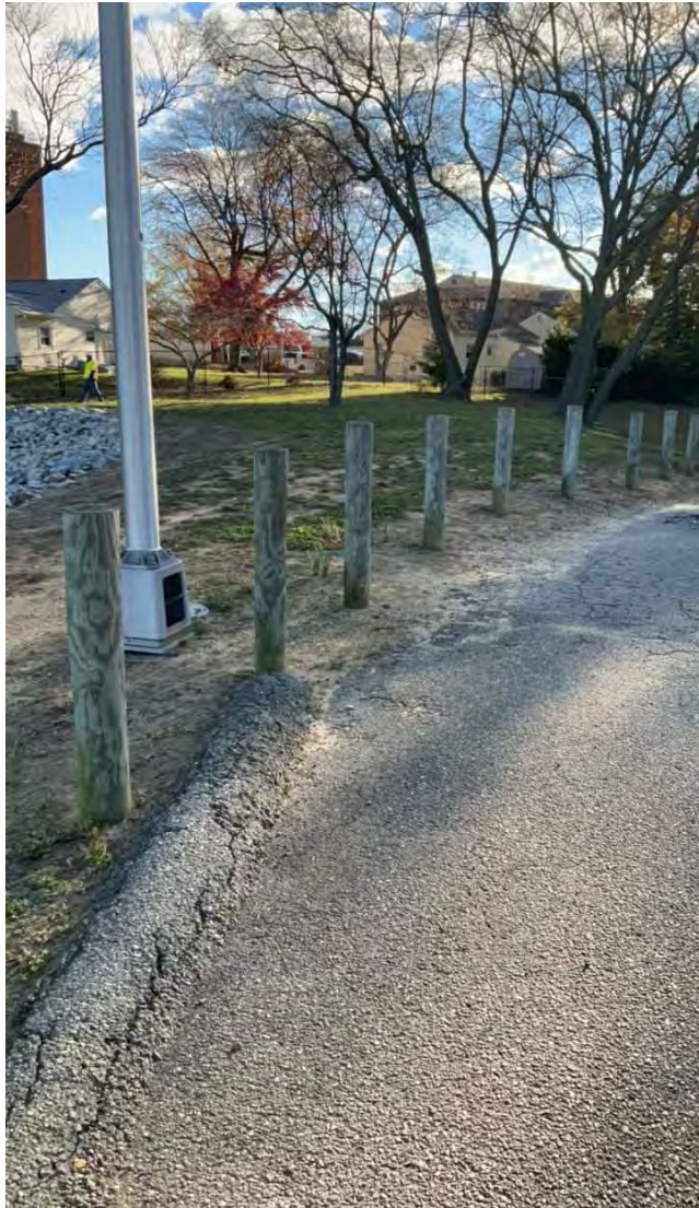
PHOTO 6: Crest of left embankment, looking east. Some bare earth, minor erosion along pavement edge.
