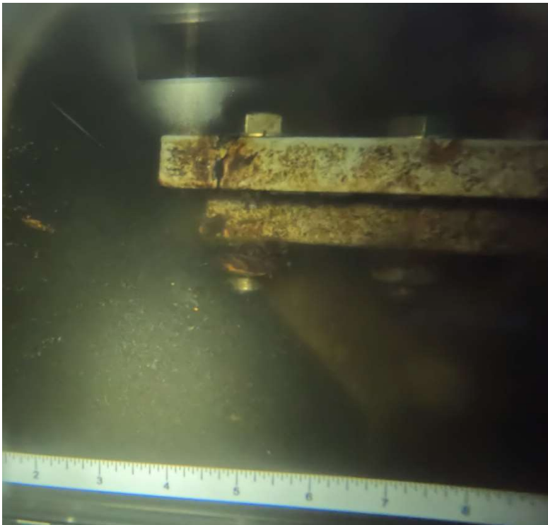
PHOTO 8: Gate frame connection
