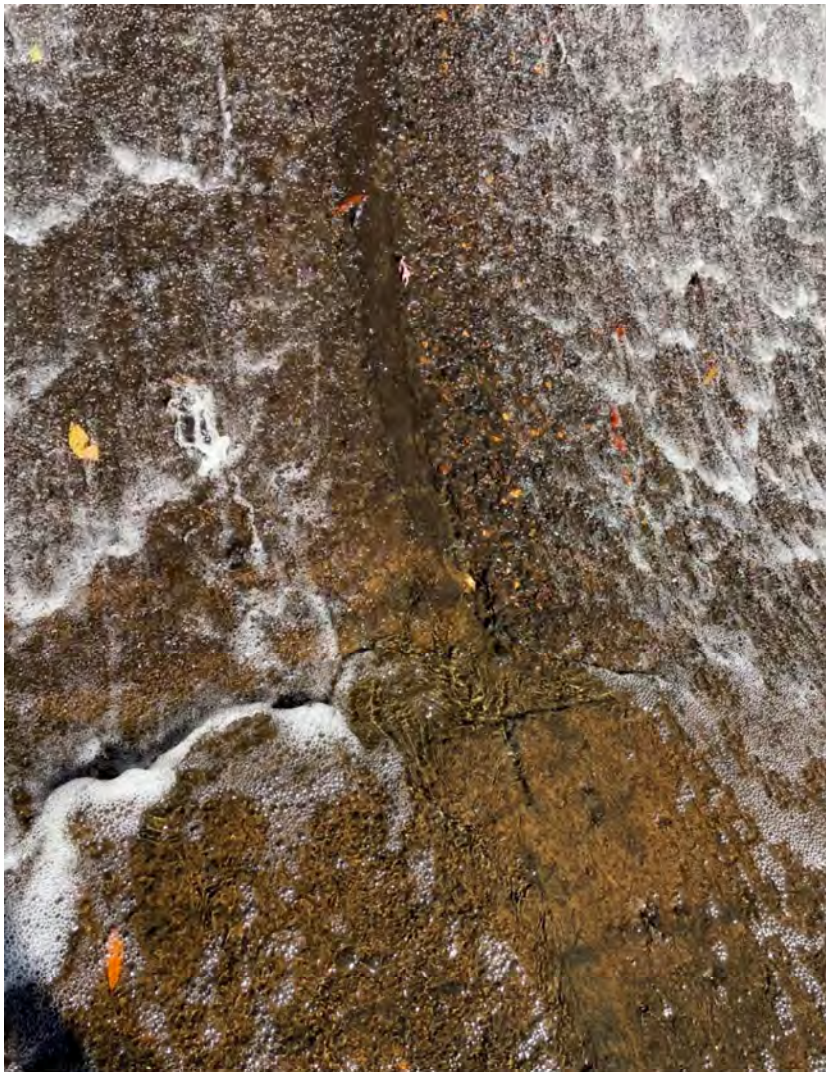
PHOTO 45: Downstream face of spillway at construction joint and prior repair.
