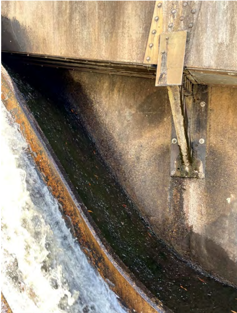
PHOTO 55: Closeup of left training wall at upstream most seep (at steel brace)
