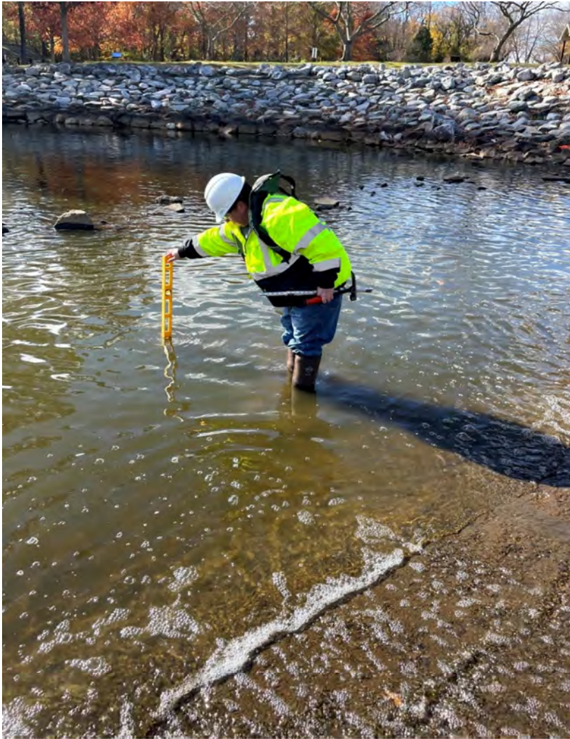
PHOTO 47: End of concrete apron, beginning of displaced riprap within stilling basin.
