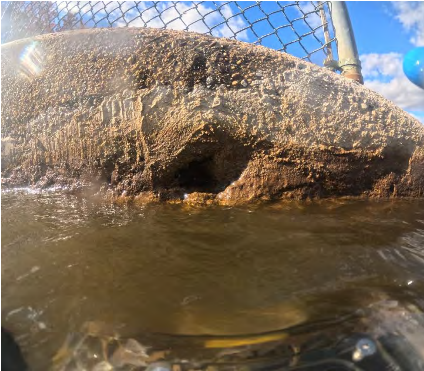
PHOTO 23: Prior concrete repair at right training wall
