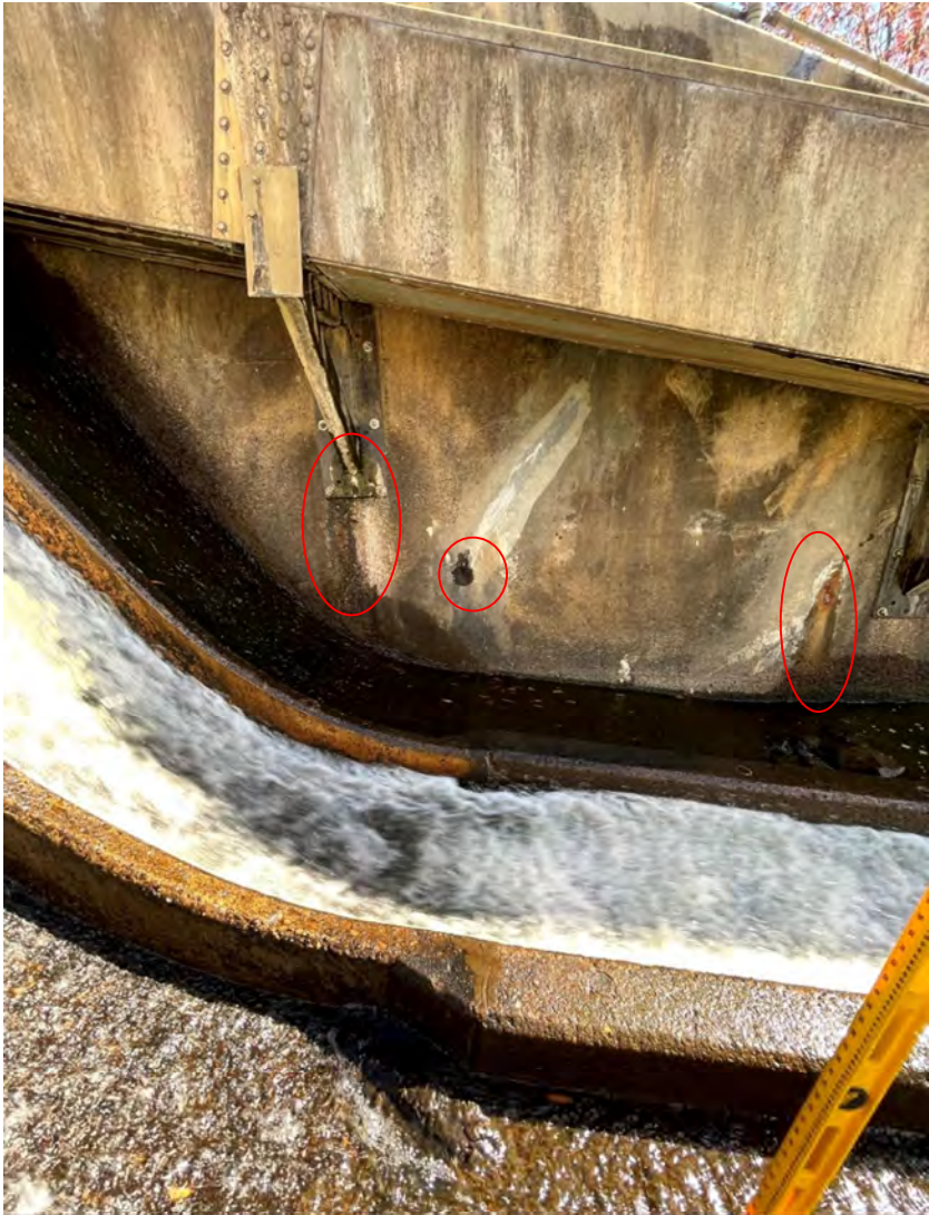
PHOTO 54: Location of seeps on face of left training wall.
