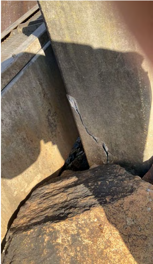
PHOTO 29: Damage at downstream end of left spillway wingwall, adjacent to fish ladder.
