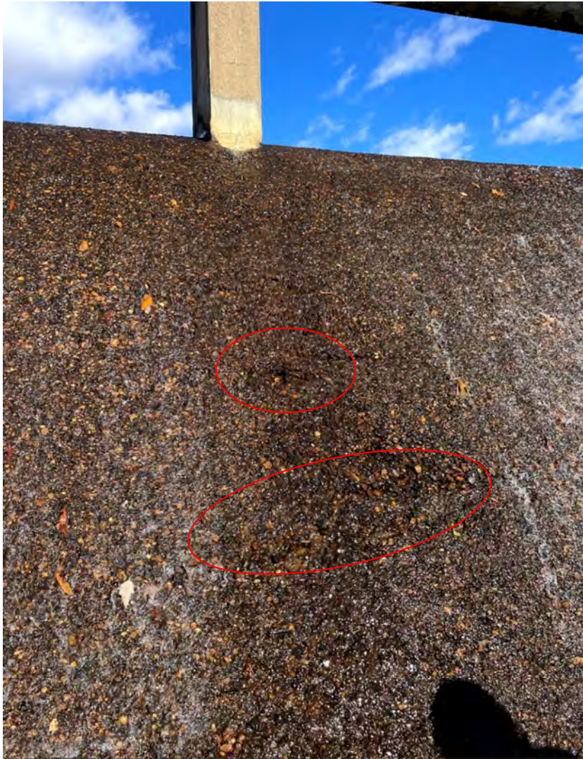
PHOTO 49: Abrasion of concrete, deeper areas of eroded aggregate sporadic along downstream face.
