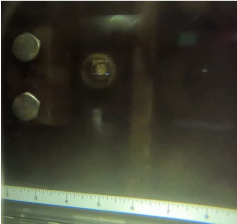
PHOTO 11: Side wedge, typical condition
