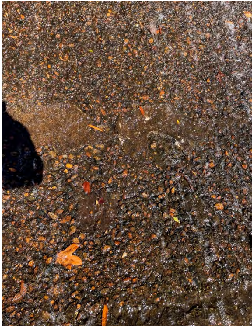
PHOTO 48: Abrasion of concrete and exposed aggregate, typical over entire downstream face of spillway.
