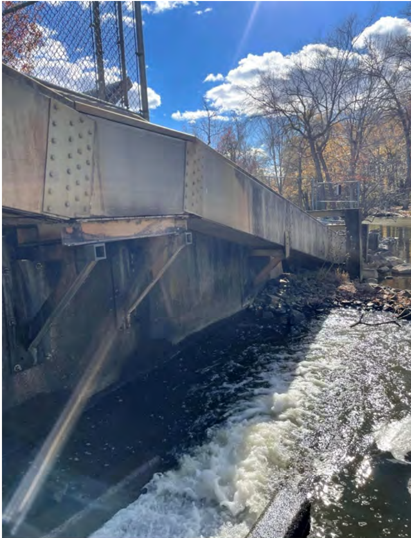
PHOTO 58: Face of left spillway training wall below fish ladder.
