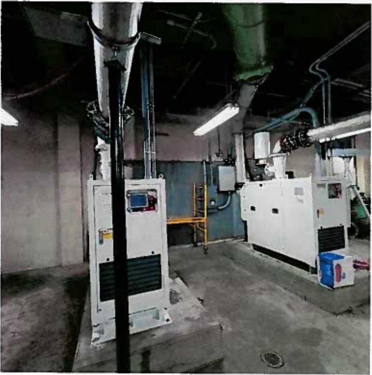
Secondary Building Basement Air Blowers
