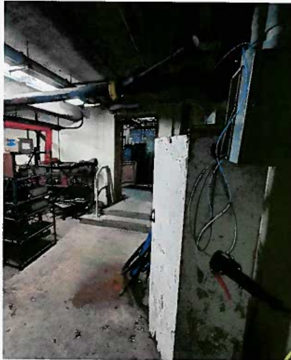
Primary building basement plumbing storage room - waste pipe leak and puddle below.
