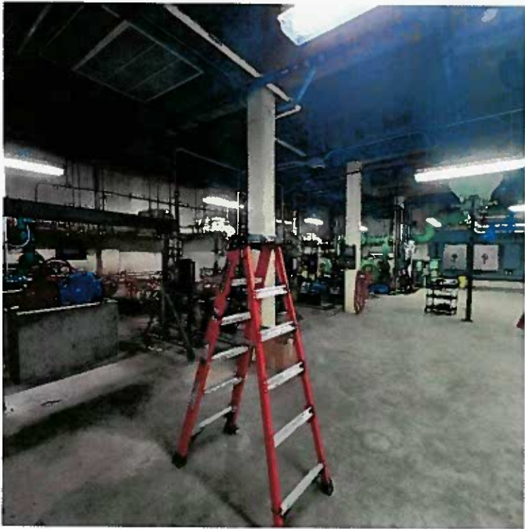
Secondary Building Basement Pumps
