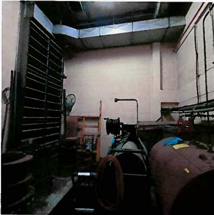
Secondary Building Main Level Air Intake Louvers and Floor Grate (Blower Make-up Air) & Generator Fuel Tank
