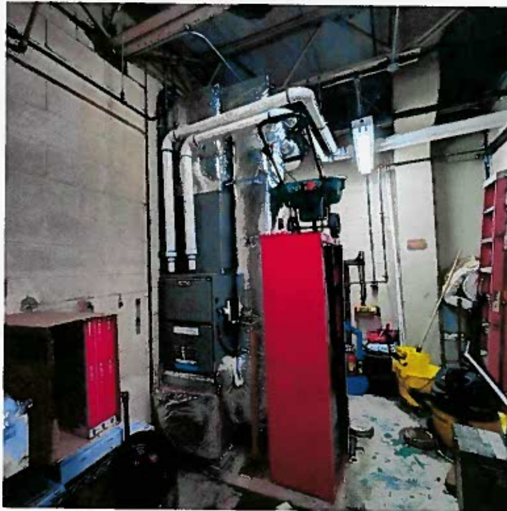
Primary Office Building Furnace/Utility Room
