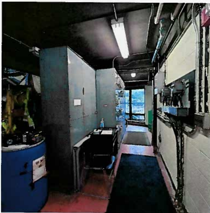
Secondary Building Main Level - Electrical Switchgear
