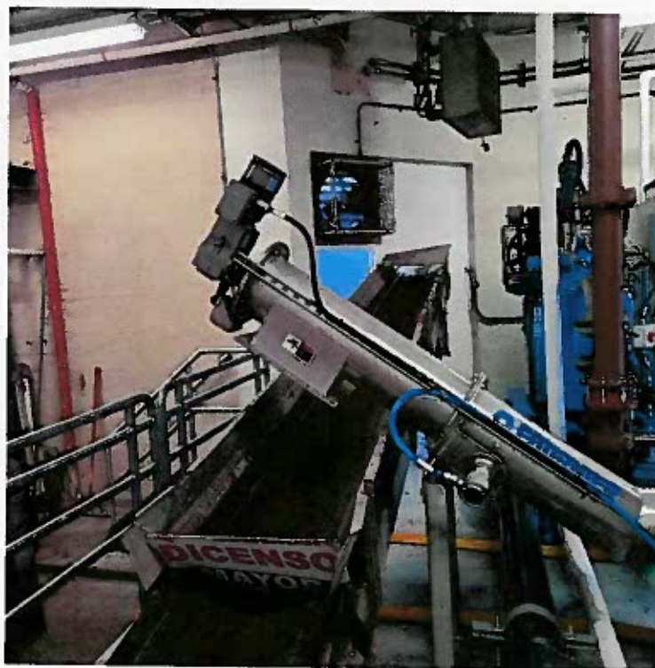
Solid Waste Conveyor to outside waste container
