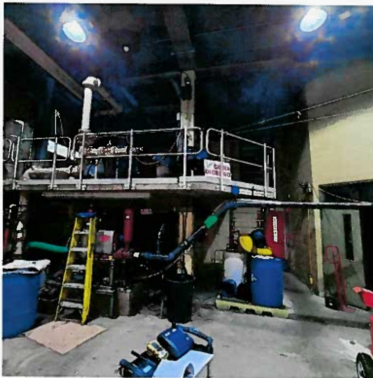
Secondary Building Main Level Decommissioned drum thickener/filter machinery
