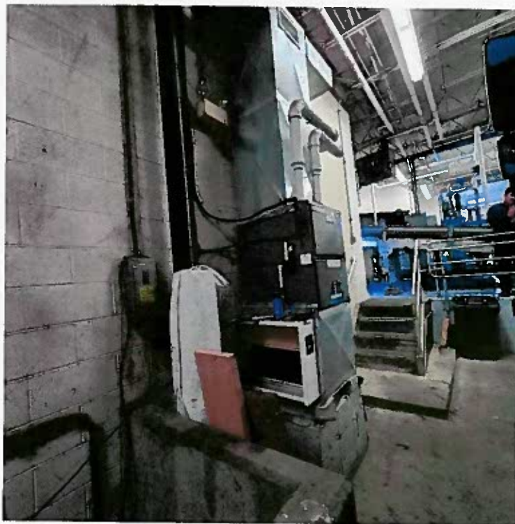
Primary Building Garage Furnace with no air filter in return air filter housing
