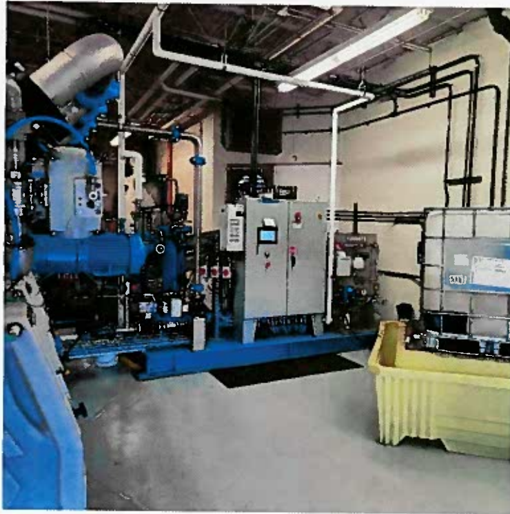
Pump Room Workspace with rainwater puddling on the floor from conveyor wall penetration.
