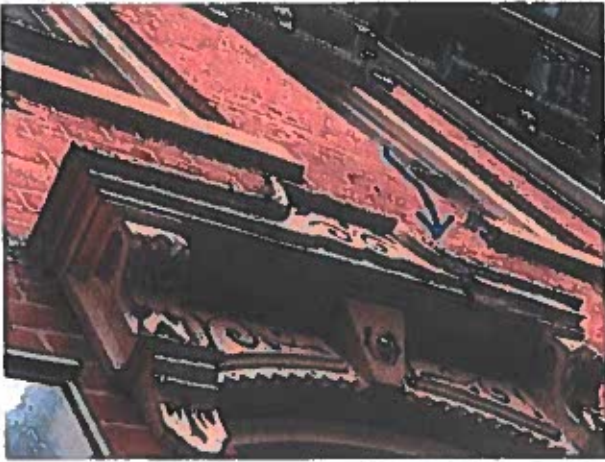
ROTTED TRIM HOOD MOULDS
