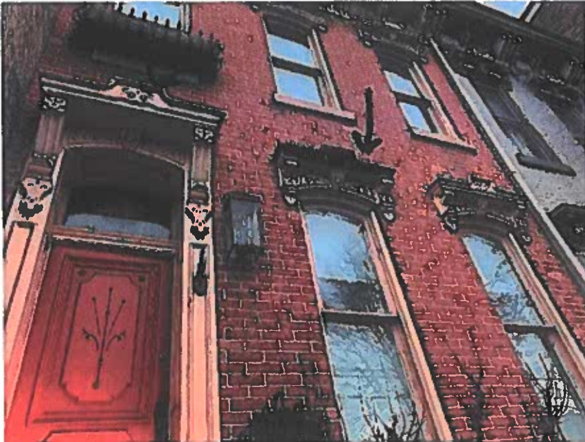
ROTTED HOOD MOULD
