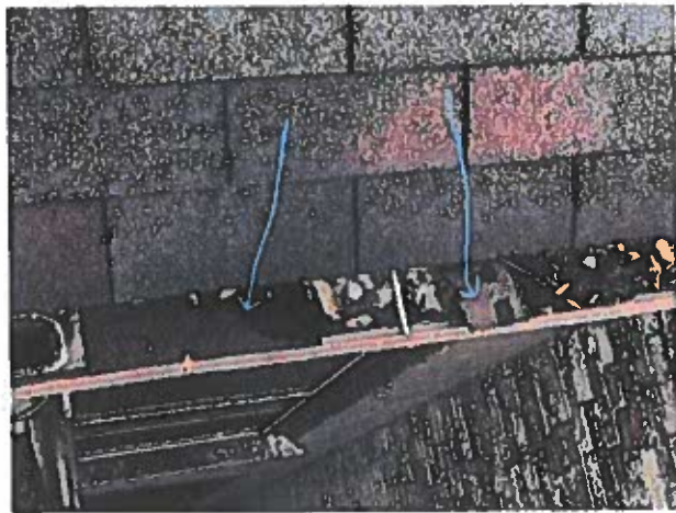
SHINGLES FALLING OFF IN GUTTER
